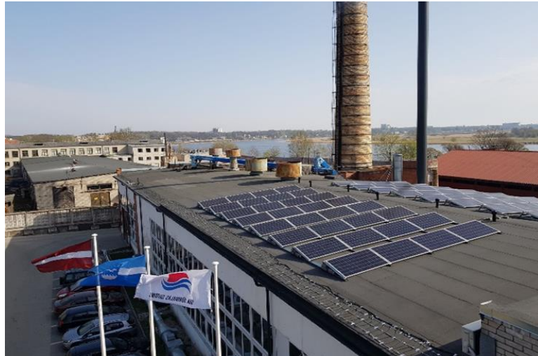
Fig. 3.3. Installed solar panels in Jurmala (Čivčiša, 2019)
