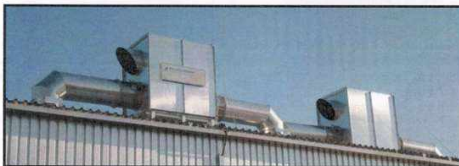
Drying kilns with heat recovery systems.
